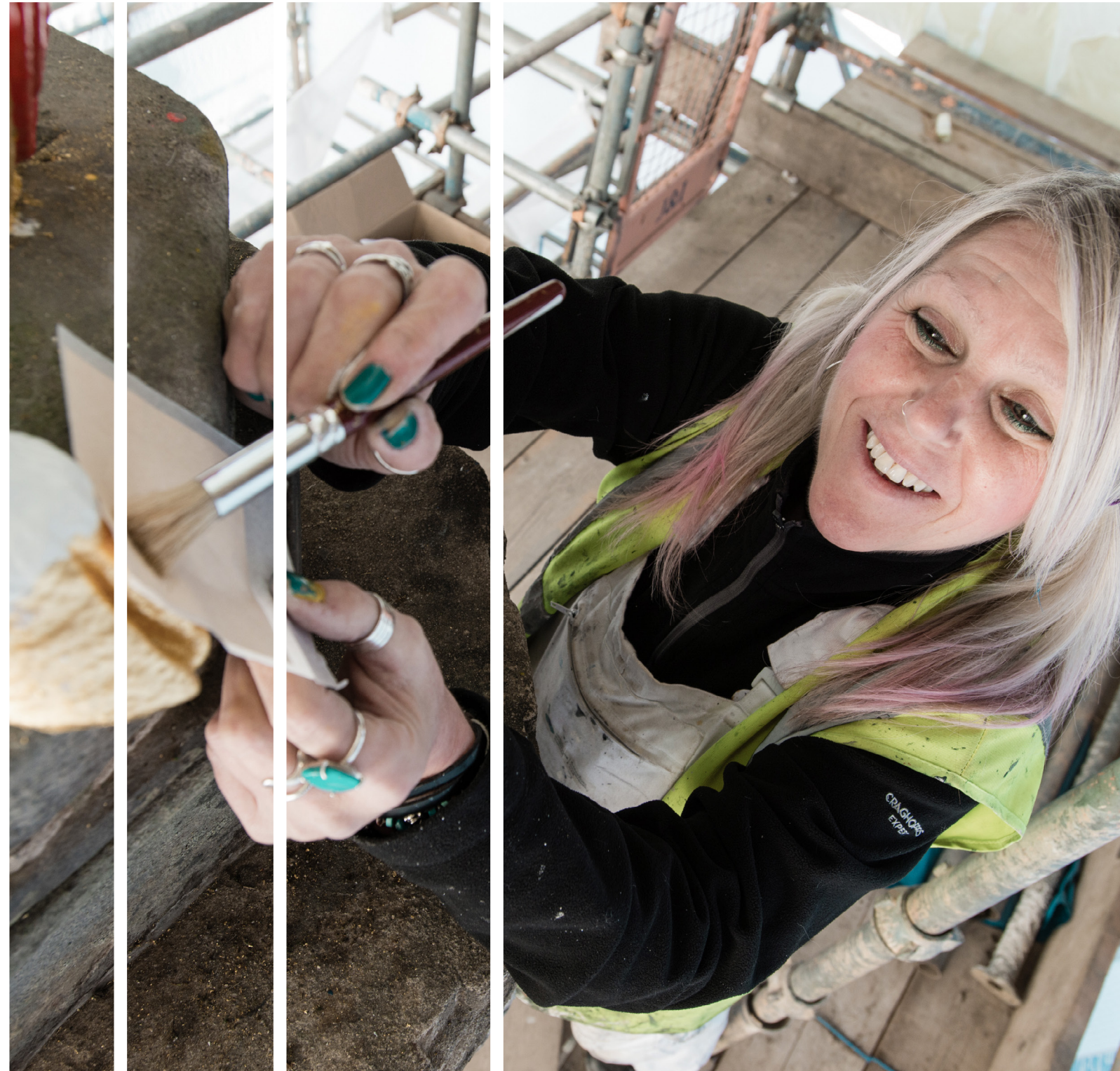
Apprentice painter, Tracey Clayton, gilding the plinth stone for the Mary Queen of Scots statue that is to be erected at Linlithgow Palace.
